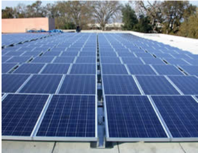
PV electricity generation
